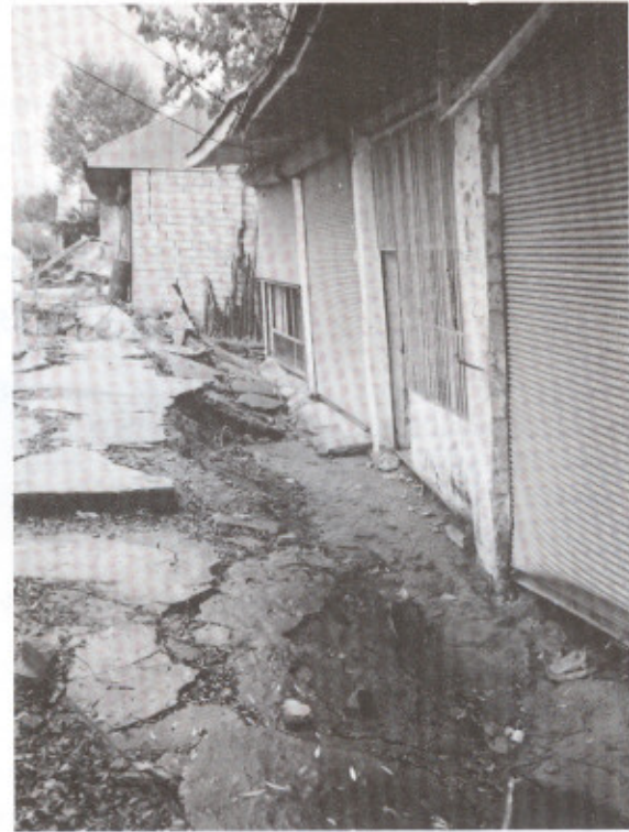
Fig. 8. Liquefaction-Induced Settlement of Single-Story Structures in Roudboneh
