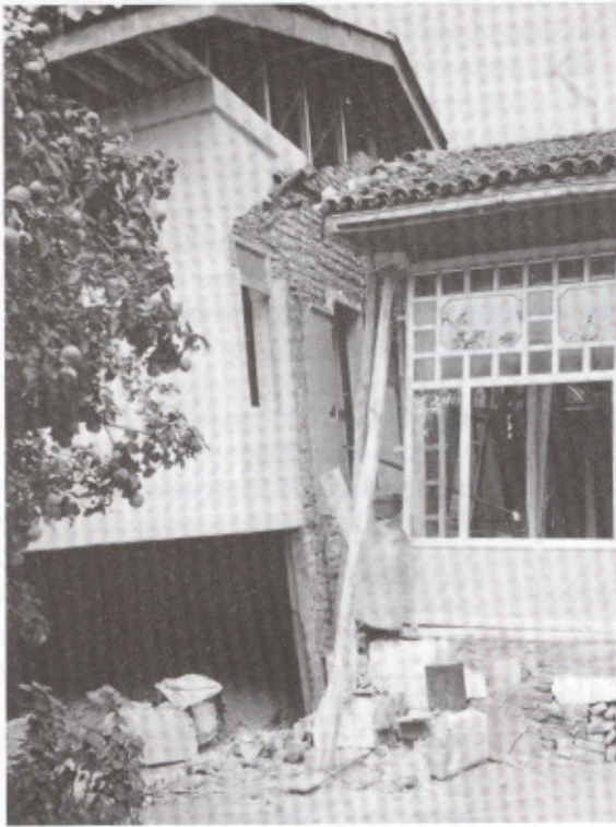
Fig. 6. Settlement and Tilt of a Building on Liquefied Sand in Astaneh-Ashrafieh
