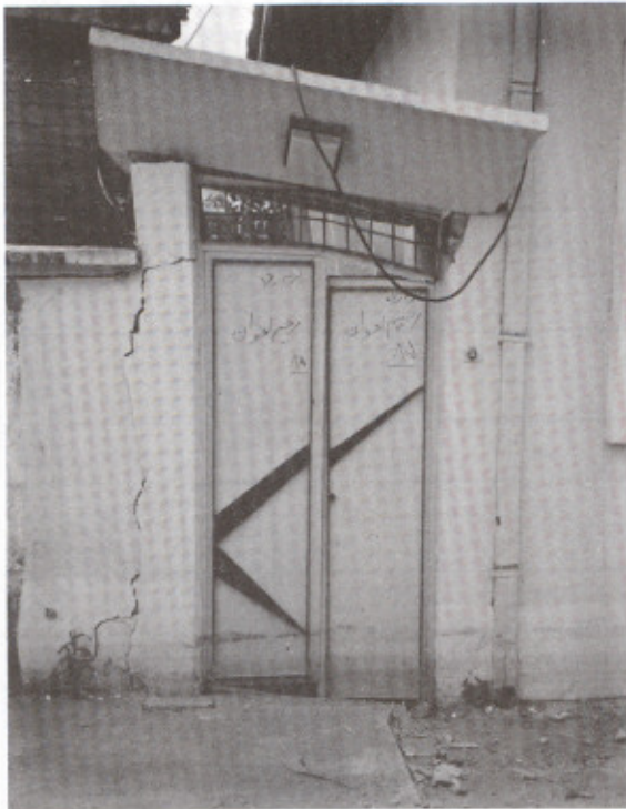
Fig. 7. Liquefaction-Induced Differential Settlement Between a House and an Adjacent Wall in Astaneh-Ashrafieh
