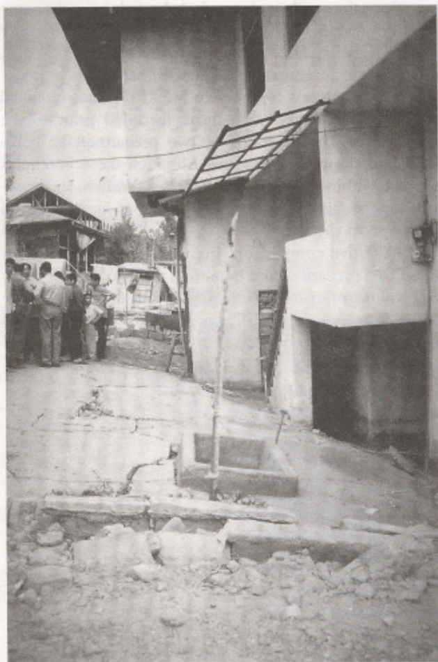
Figure 8. Liquefaction-induced settlement (70 cm) of a two-story building in Astaneh-Ashrafieh.
