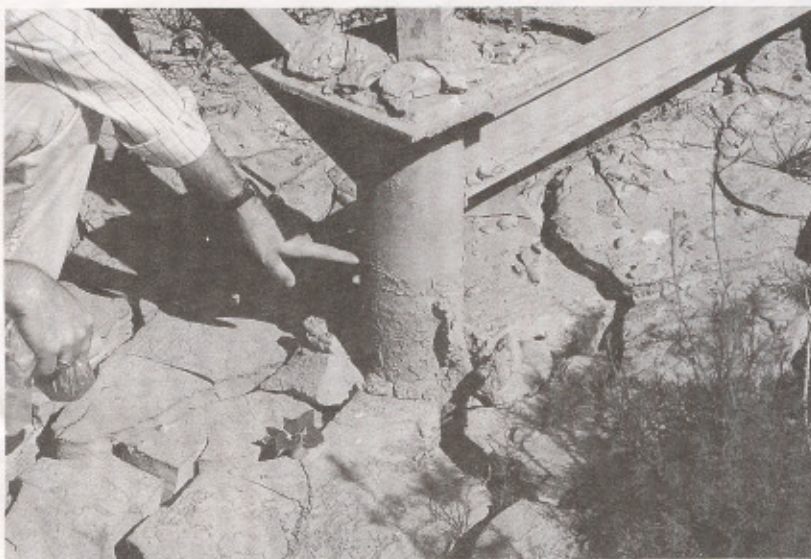
Figure 29. Photograph depicting ground settlement around the 15-cm-diameter pipe piles of the trestle.
