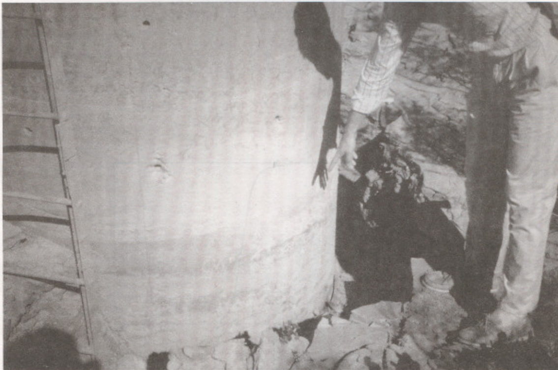
Figure 24. Photograph showing settlement and permanent lateral displacement of the ground around the Bala-Bala bridge pier.
