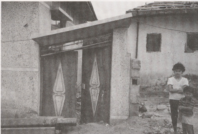
Figure 7. Photograph illustrating liquefaction-induced building settlement in Astaneh-Ashrafieh. (Note the distorted door-jamb depicting the magnitude of the building settlement.)
