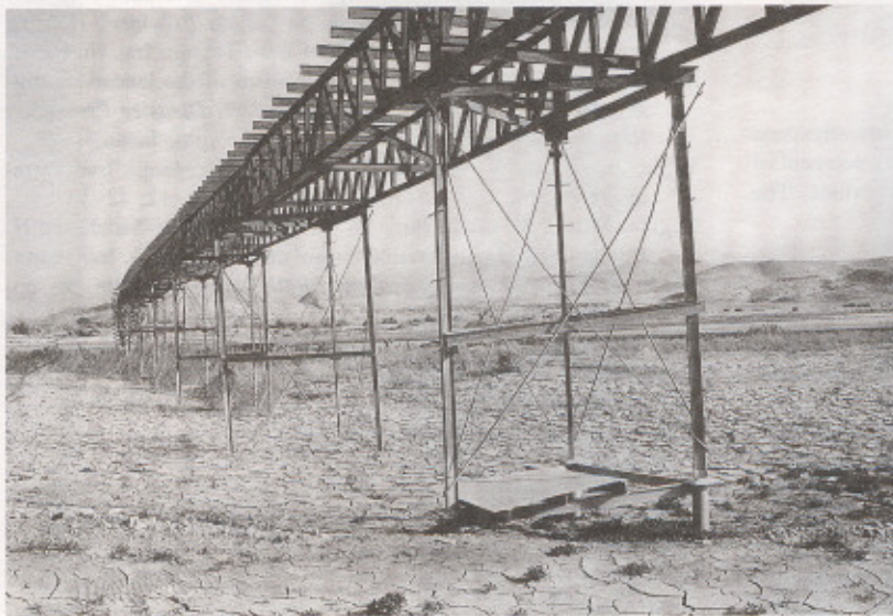
Figure 28. Photograph of a trestle founded on liquefied sand.
