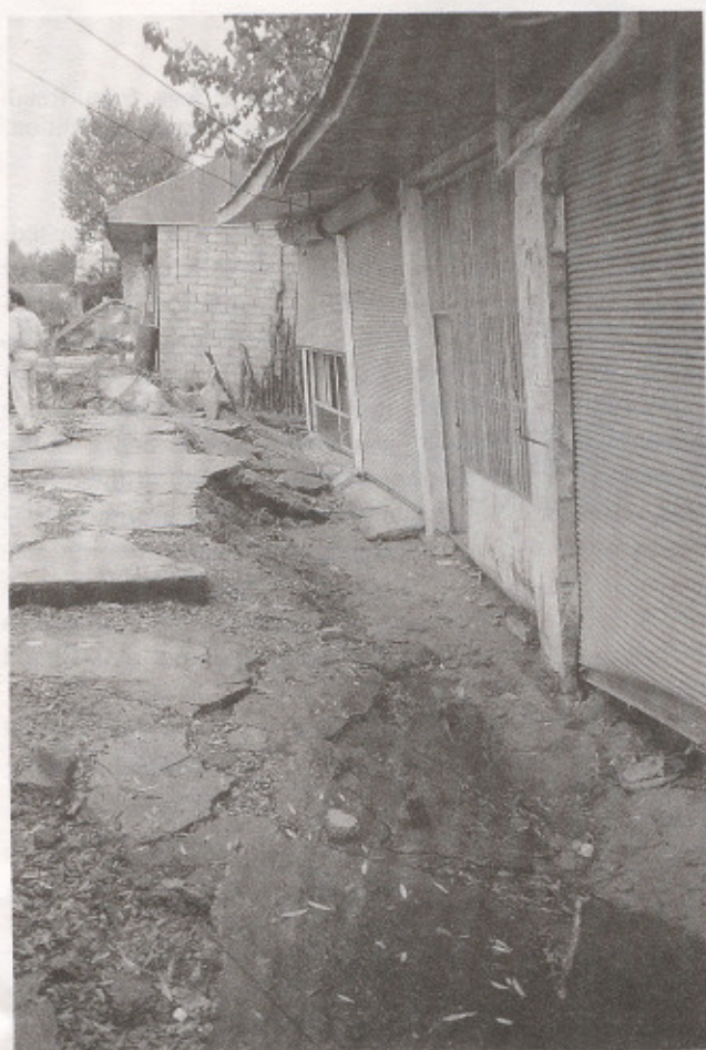
Figure 15. Photograph depicting liquefaction-induced settlement (60 to 70 cm) of a row of stores in Roudboneh.
