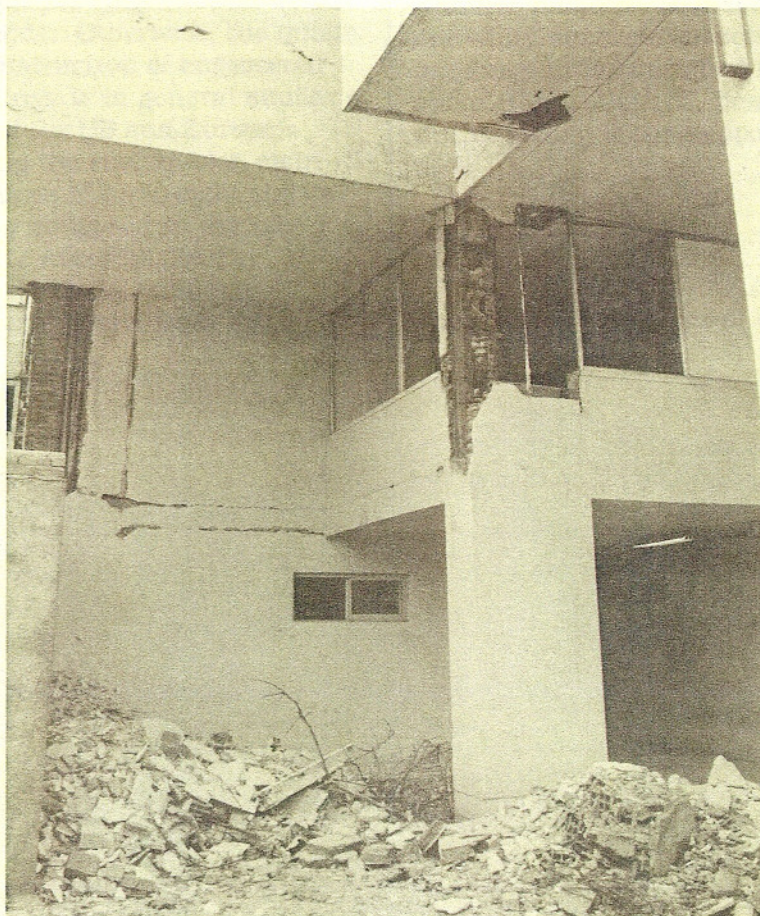
Damage to exterior of the hotel Bozorge Guilan
