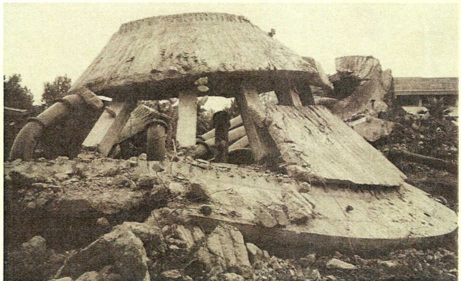
Empty R/C elevated tanks developed cracks, while full tank collapsed.
