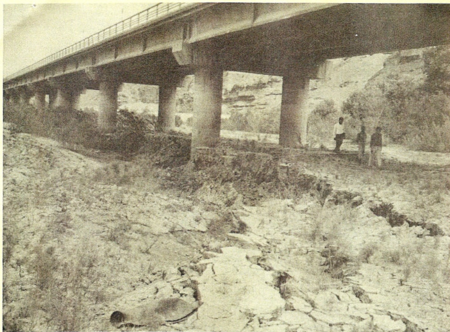
Soil liquefaction and sand boils under Bala-Bala bridge.
