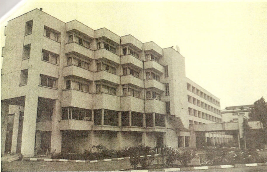
Damage to exterior of the hotel Bozorge-Gullan.
